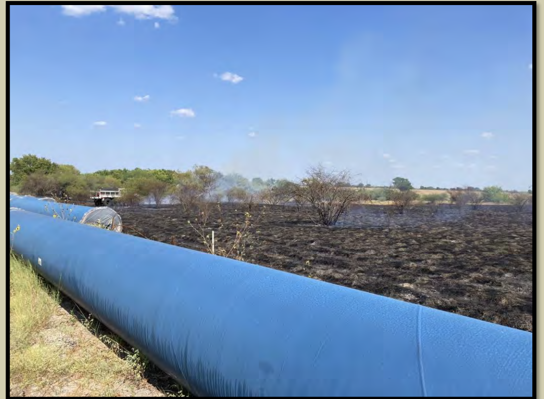
FIRE NEVER CROSSED PIPE
