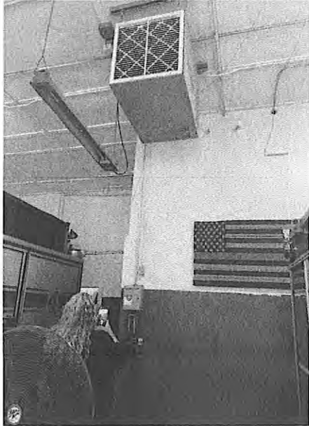
Existing air scrubber
