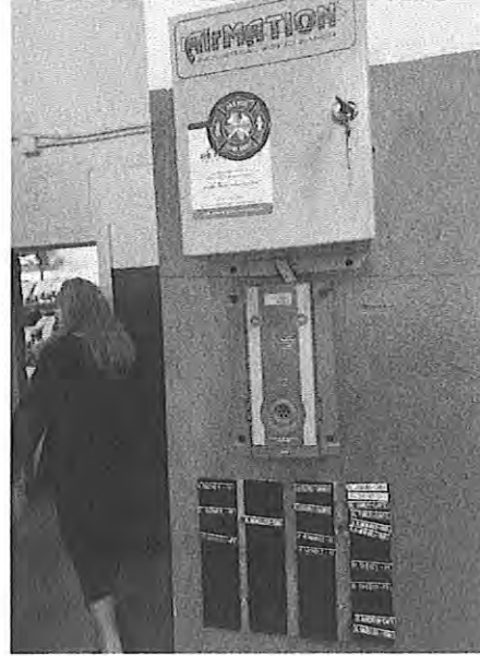
Existing air monitoring system
