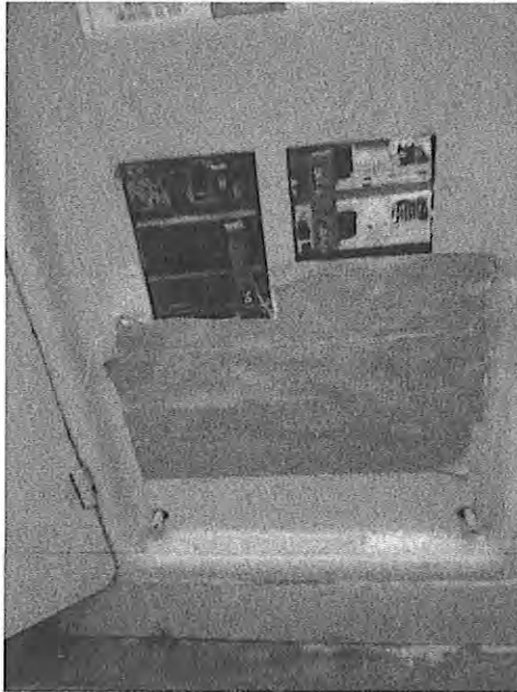
Panel in poor repair...duct tape is not always the universal solution
