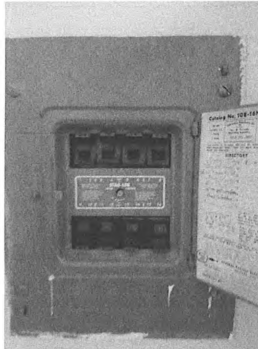
Federal Pacific sub-panels
