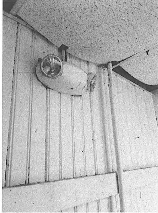
Existing Emergency Light
