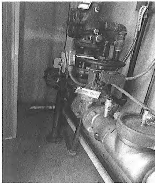
Picture of typical fire sprinkler system riser
