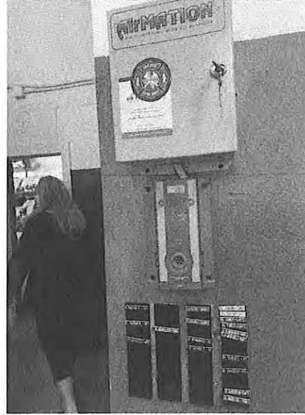
Existing air monitoring system
