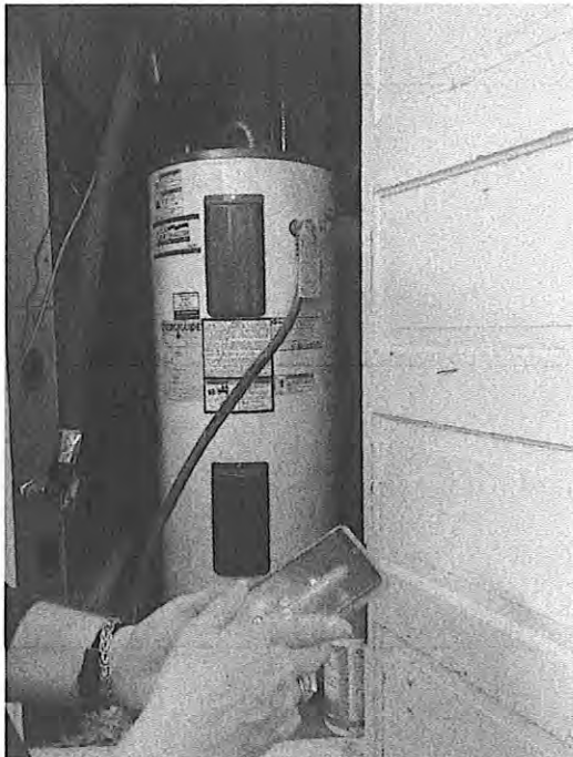
Existing water heater
