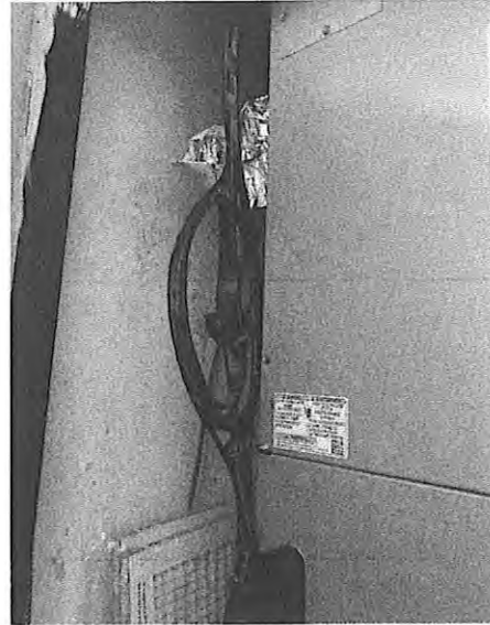
Existing System #2 AHU
