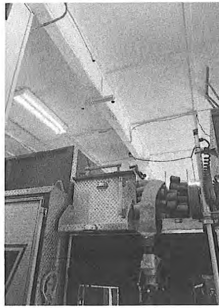
Location of damaged heater
