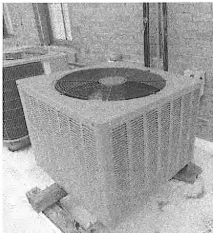
Existing System #1 CU
