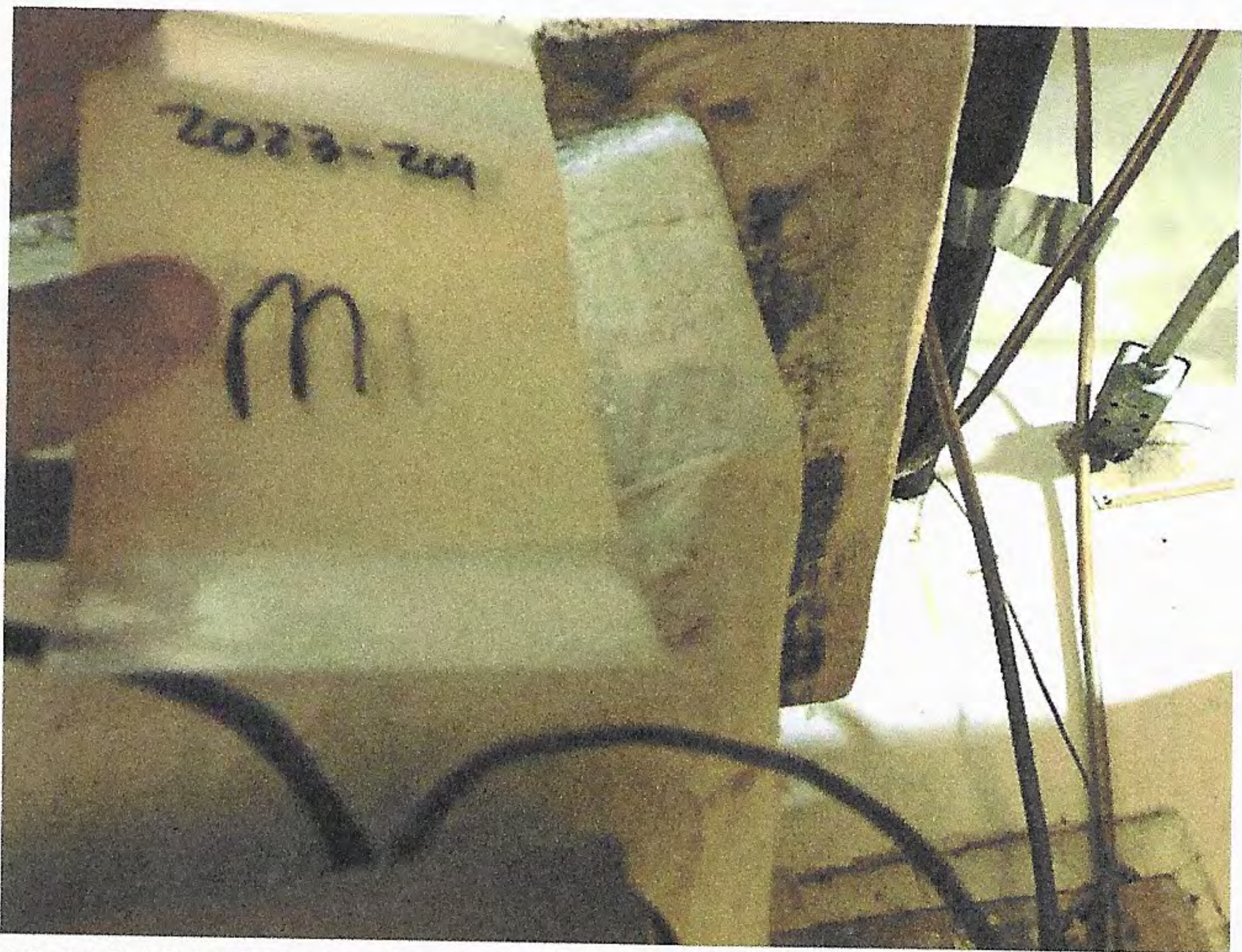
M-M2 HVAC Duct Sealant Mastic
