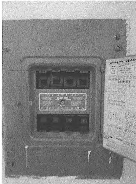
Federal Pacific sub-panels
